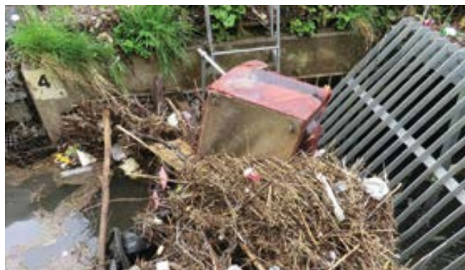
locked up culvert
